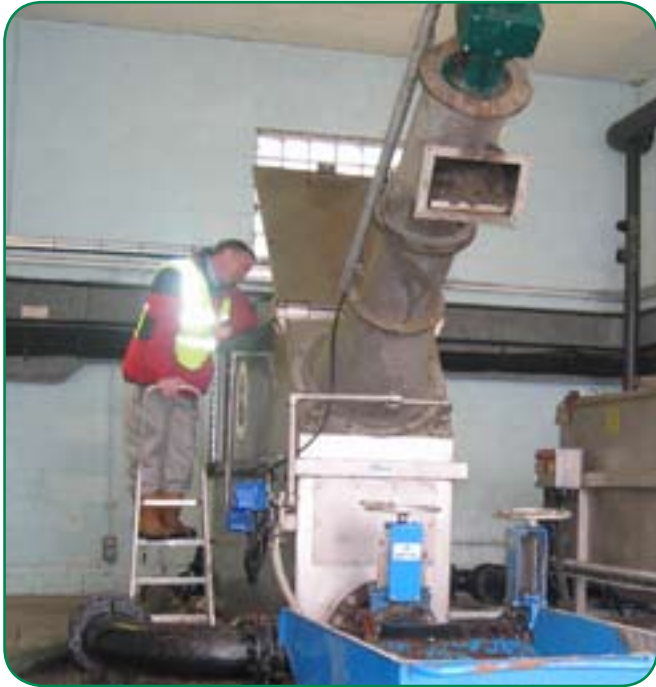
Honey Monster at a sludge screening plant in the UK.
