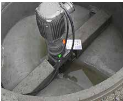
A 3-HYDRO-C Sewage Shredder with submersible Motor at a Veterinary Clinic
