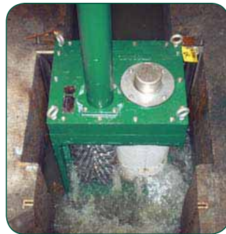
A model CMD replaced an old comminutor.
