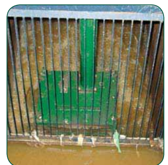
Channel Monster with overflow bar rack.
