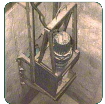
Channel Monster installed in pump station with guide frame.
